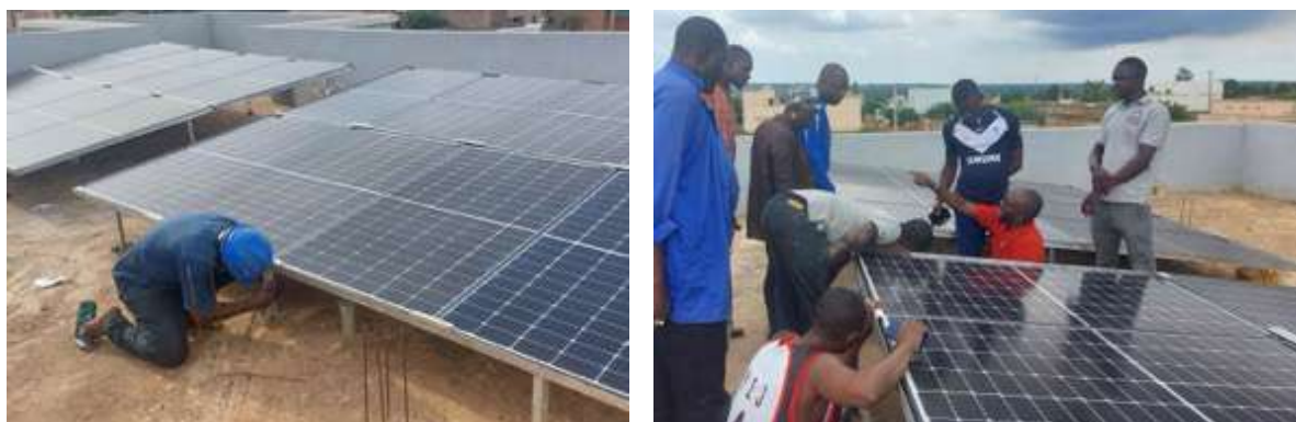
Photo 2: Solar back-up installations in the LRP
